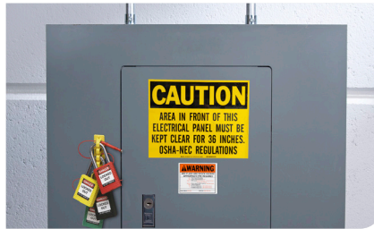
Panel and Enclosure ID
