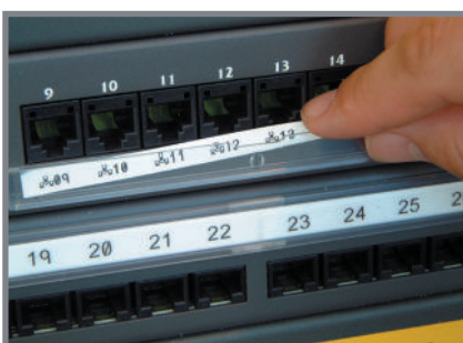
Punch Block & Patch Panel Labels
